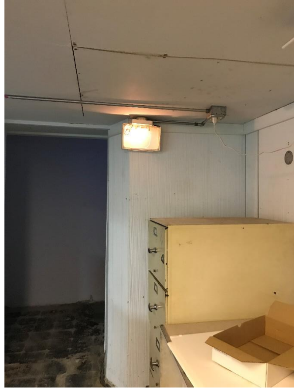
Repair Exit sign to meet WI Building code
