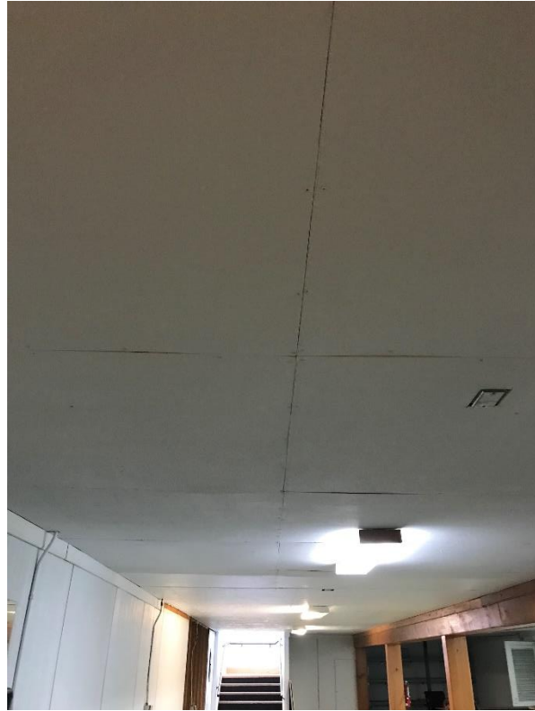
Update lighting & ceiling to meet ATCP code
