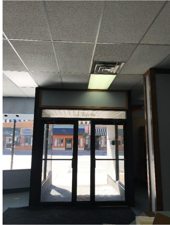
Install Exit sign to meet WI Building code
